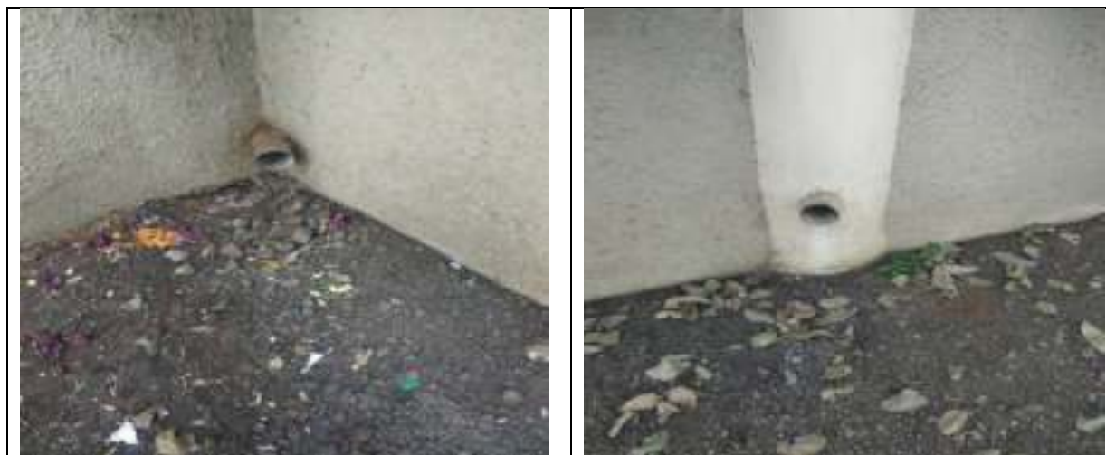
Fig 2. Rainwater harvesting system installed in the campus
